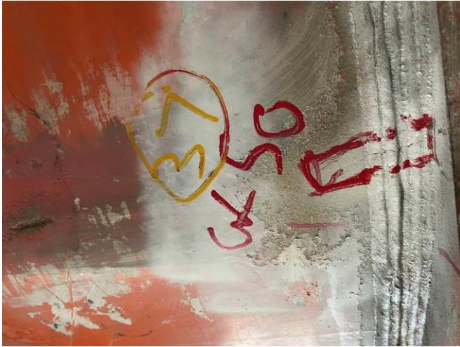
PHOTOGRAPH NO. 37 – EXTERNAL STICK TYPICAL VIEW OF DEFECT #37
